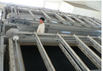
Treatment plant waiting for wastewater
