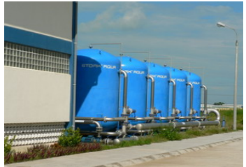
The water treatment plant for the industrial park
