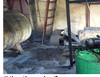
Oil spilt on the floor
