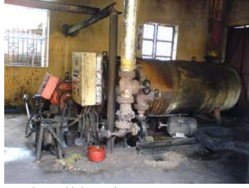
In the oil heating room
